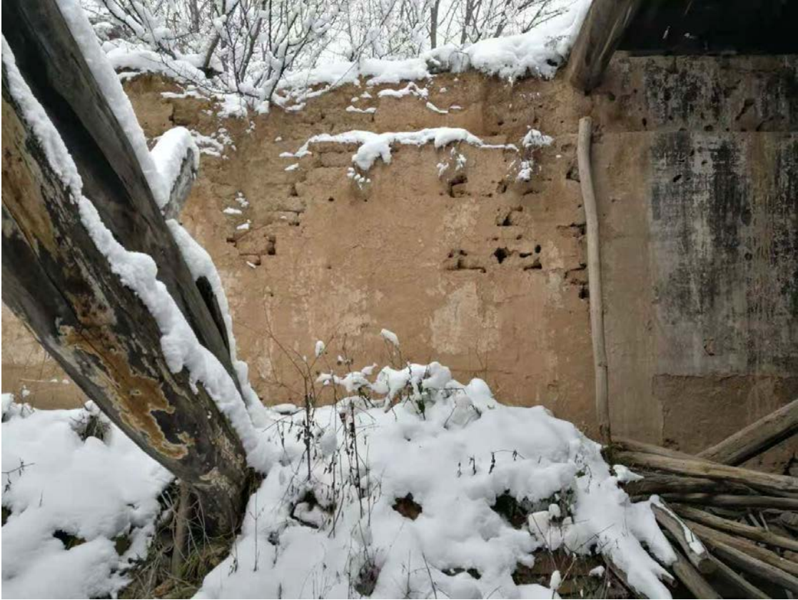
Figure 7. The roof collapsed in the main room, Zhangzhaigou
