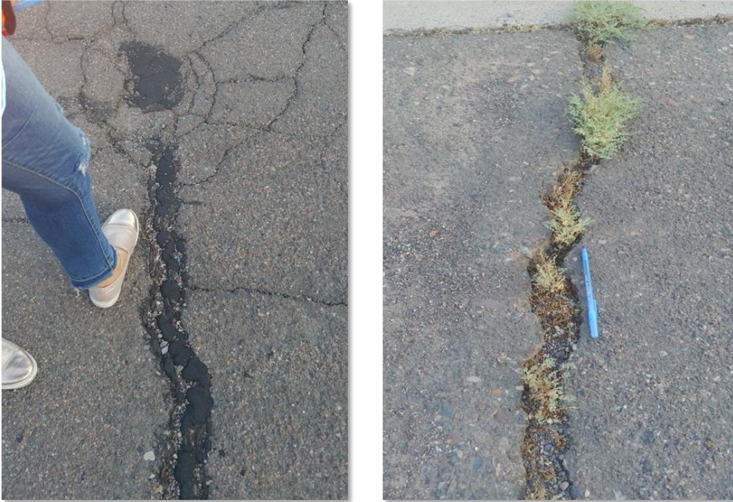
Figure 7- Crack Sealant Failure in Adhesion and Cohesion in a Parking Lot
