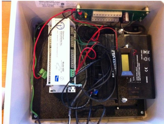
Figure 3.2 Photograph of the Data Logger and Battery Inside Containment Box
