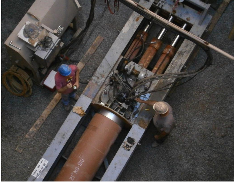
Figure 3.5 Power Pack & Data Dolphin Containment Unit Configuration for the BM Pusher During Phase 3
