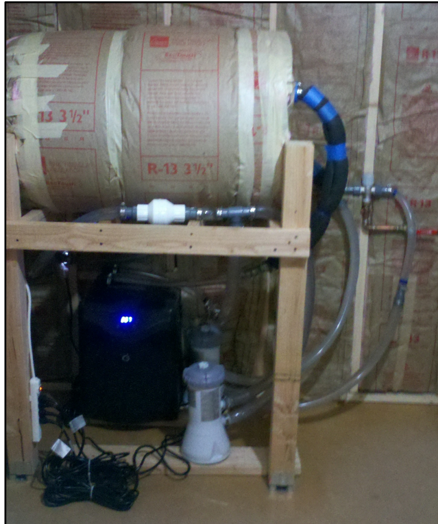
Figure 16. Cold-Water Storage Tank and Chiller.
