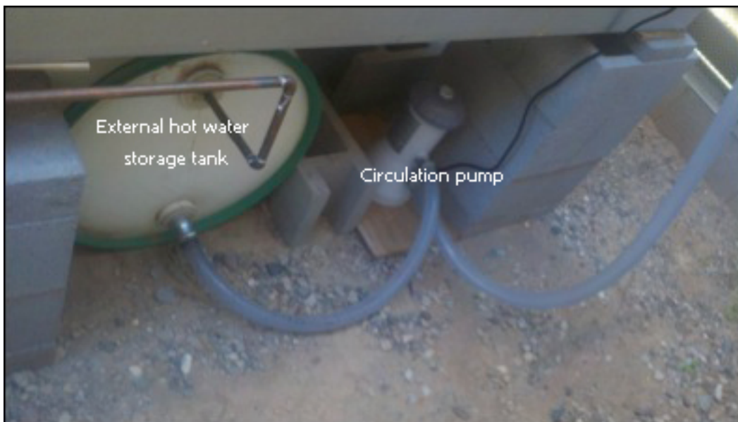
Figure 14. External Hot-Water Storage Tank and Circulation Pump.
