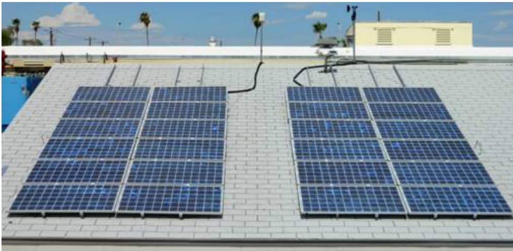
Figure 3.1 Side-by-Side PV Array
