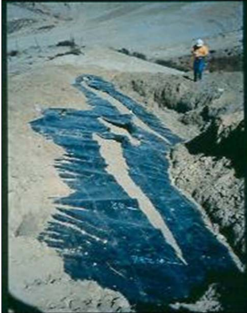
Figure 1-3 Tear in geomembrane liner system, Cell C, Chiquita Canyon Landfill after 1994 Northridge earthquake (photo courtesy of Calif. EPA, Integrated Waste Management Board)
