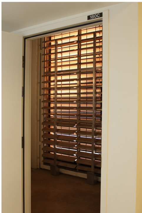
Figure B6: Intake Rooms with Louvers Open
