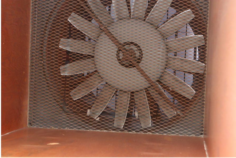
Figure B8: Main Fan
