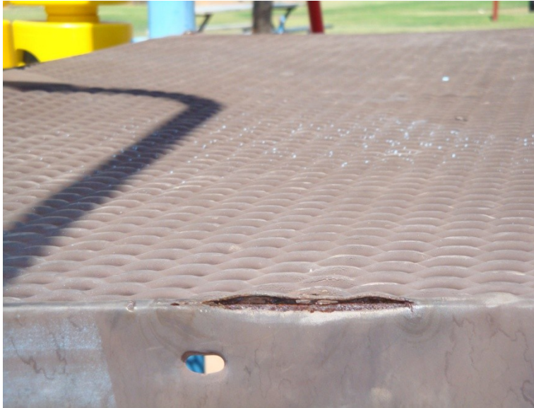
Figure 4: Rusted edge on platform
