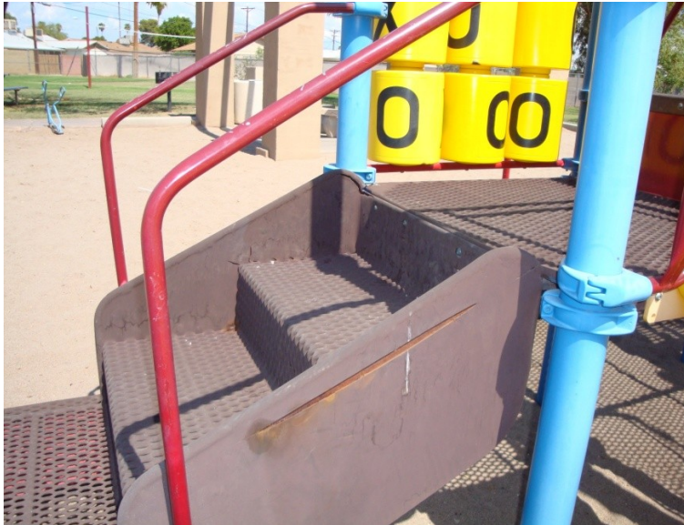
Figure 2: Rusting steps on playground
