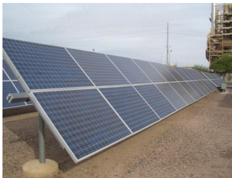
Figure 11. Photograph of OPV2A modules
