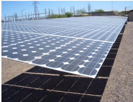
Figure 9. Photograph of OPV1A modules
