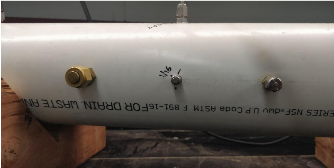
Fig 2: 1/4 , 1/16 and 1/8 inch leak
