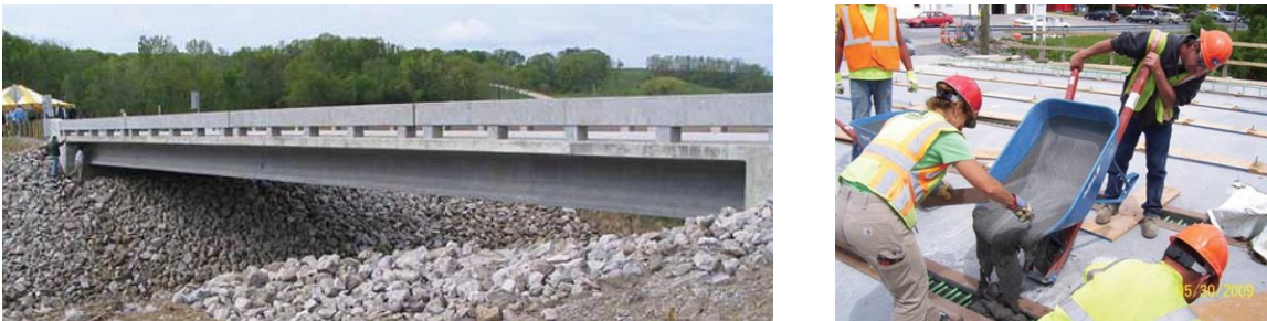
Figure 2-8: (a) The first UHPC bridge constructed in the U.S (in Wapello County, IA), (b) casting of longitudinal connections between deck-bulb-tee girders (Route 31 Bridge, Lyons NY). Both figures courtesy of FHWA.
