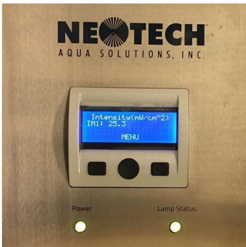
Figure 9. Close-Up view of D222 UV device control box
