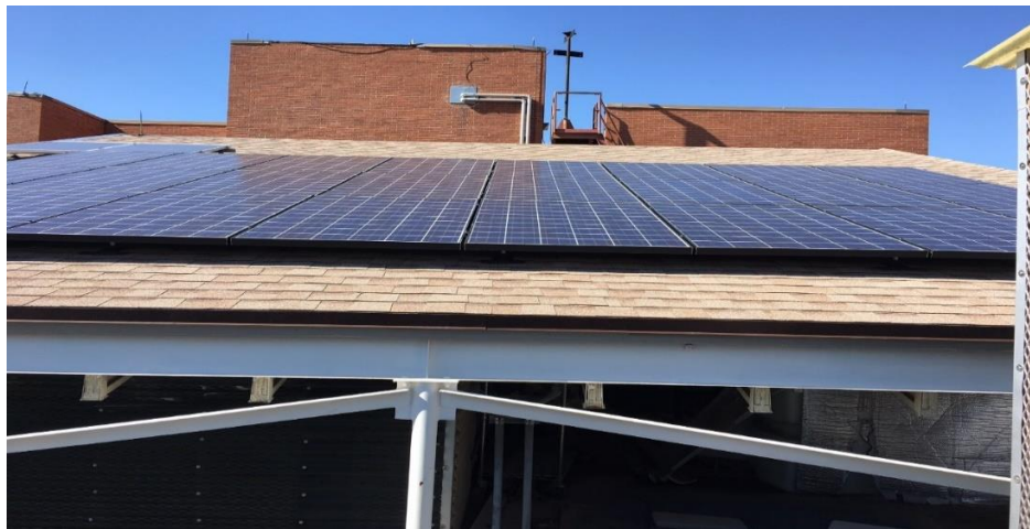
Fig. 2.1. Polycrystalline Solar Panels Rooftop ERC
