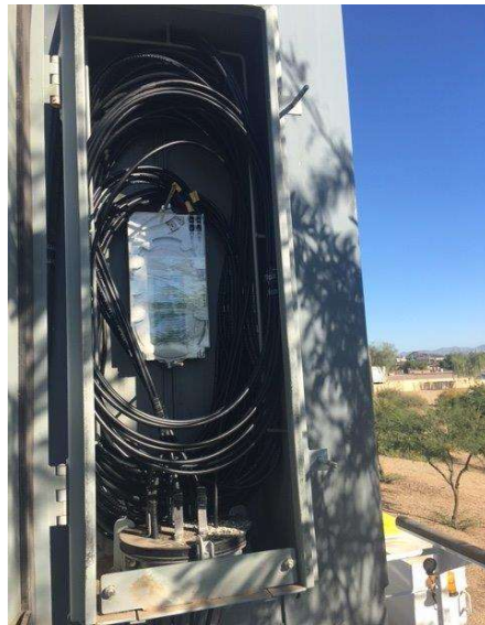
Figure 3-2 Splice box on riser pole P30
