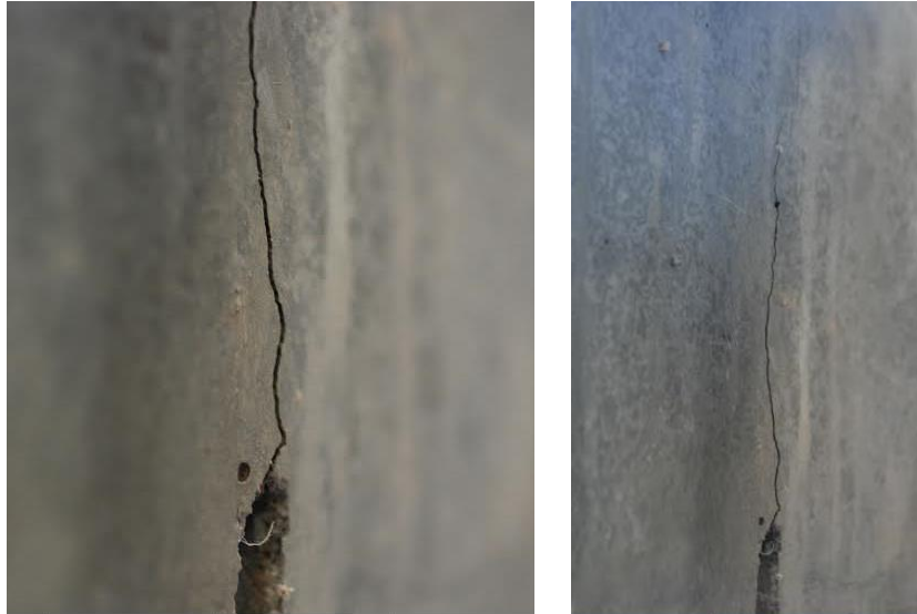
Figure 1: Crack propagation of fiber reinforced concrete under sustained loads
