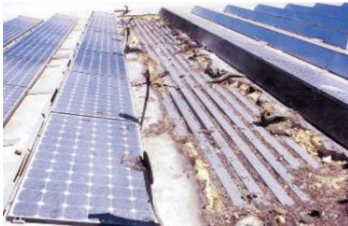
Figure 1.4 Fire Hazard in a 383 kW PV Array in Bakersfield, California in 2009. [34]
