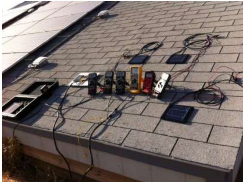
Figure 8.1 The setup of testing different solar irradiance sensors
