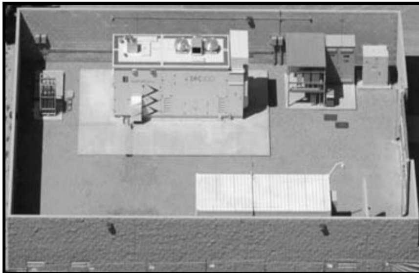
Figure 2.5 Commercial fuel cell running on natural gas at ASU east campus [24]
