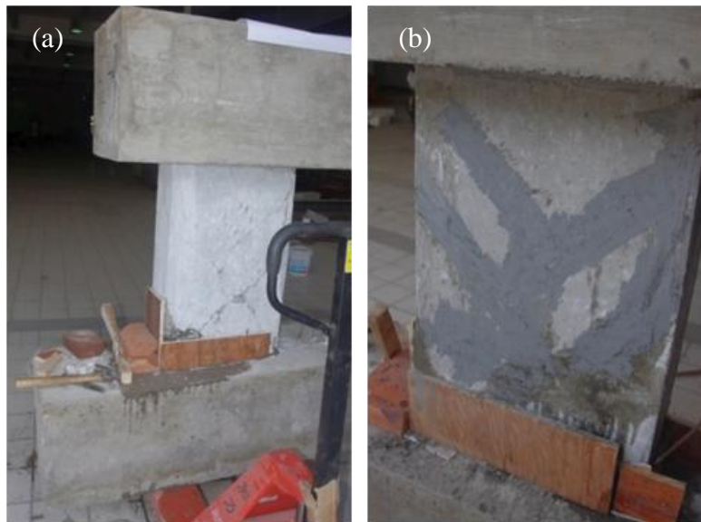
Figure 7.3.1.1. Repair of the damaged RC shear wall: (a) grouting; and (b) crack epoxy injection [144] 20
