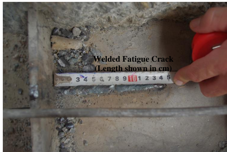
Figure 6.2.2.2. The welded fatigue crack on the encased steel section, crack length shown in centimeters
