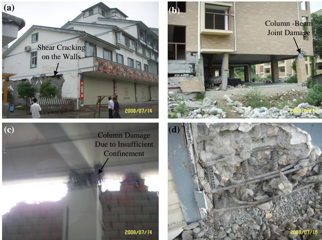
Figure 1.1.2. Structural damages caused by earthquake (Wenchuan, China, 2008): (a) seismic induced shear cracks on masonry walls; (b) column-beam joint damage; (c) column damage (top); (d) column damage (bottom) 2
