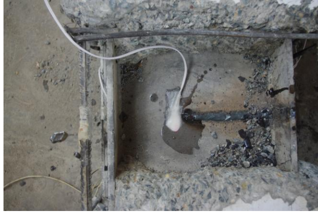
Figure 6.2.3.2. Strain gauge installed at the fatigue crack tip to monitor the weld fracture
