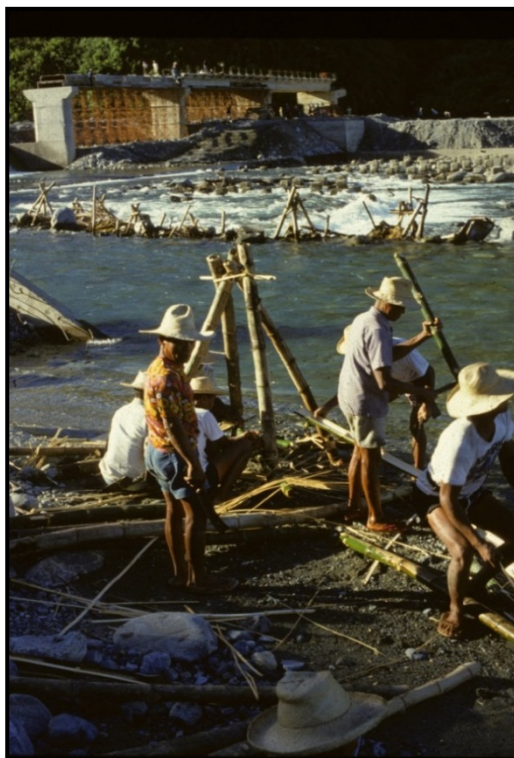
Figure 3. Zanjera San Marcelino farmers re-building bamboo, stone and brush dam (INIP Madongan Dam under construction in background). Source: Photo taken by Ruth Yabes, 1985.
